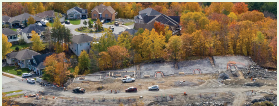
Site preparation for Phase 2 of the Hall Construction subdivision Thunder Creek began in 2019. Shortly after the Housing Summit, the owner "up-zoned" the subdivision to medium density residential. The subdivision is located at the end of Winnifred Avenue behind the Parry Sound High School.
